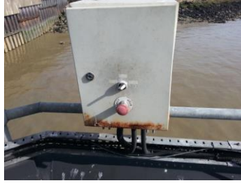
Emergency & Two-Way Switch
