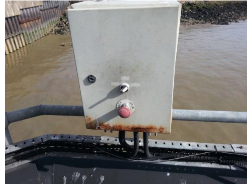
Emergency & Two-Way Switch
